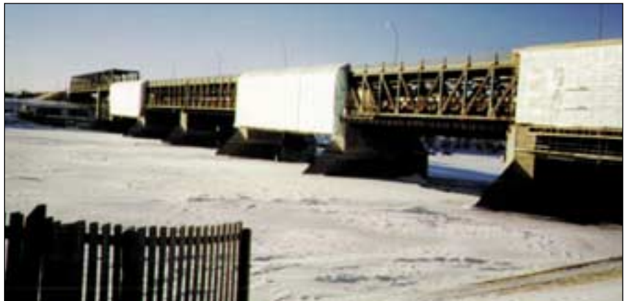
Fig. 2 - Containment structures for blasting, metallizing, and climate control throughout job. Photo courtesy of PWGSC and Wardrop Engineering
